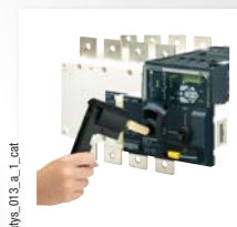
Emergency manual operation
